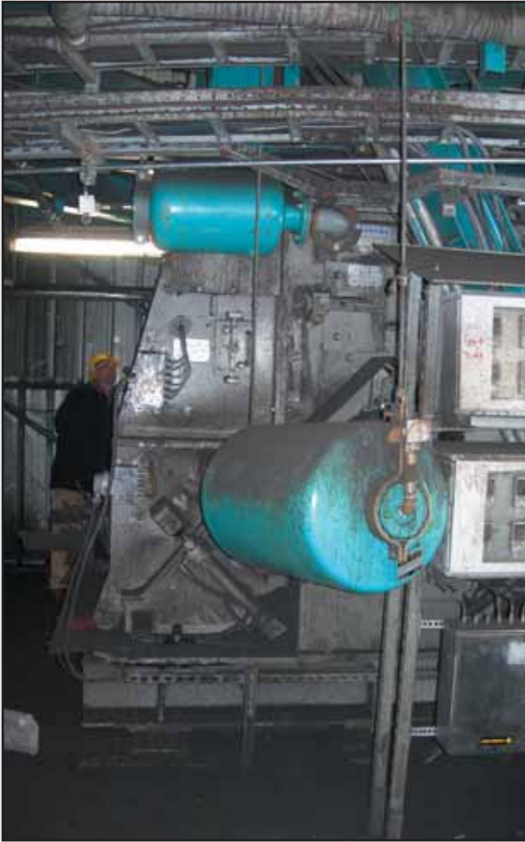
CRUSHER SURFACE-THERMAL POWER PLANT
