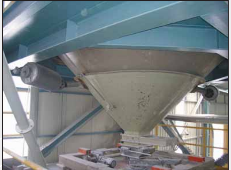
END PRODUCT SILO-MINING FACILITY
